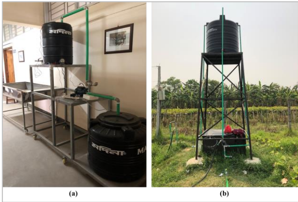
Fig. 4. Pump automation system.
